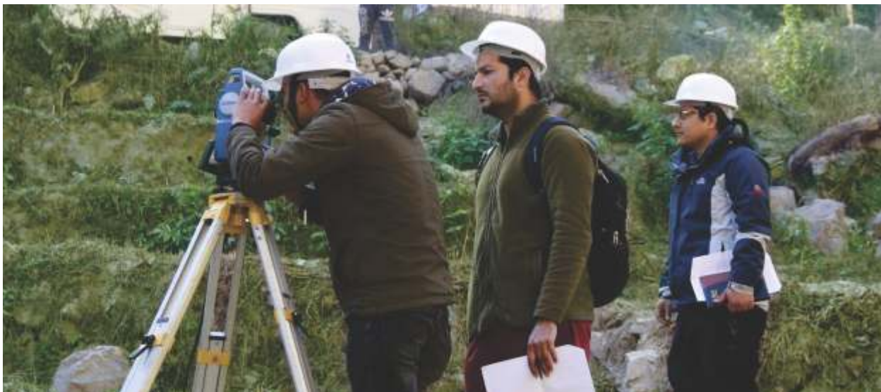
Survey of Transmission Line
