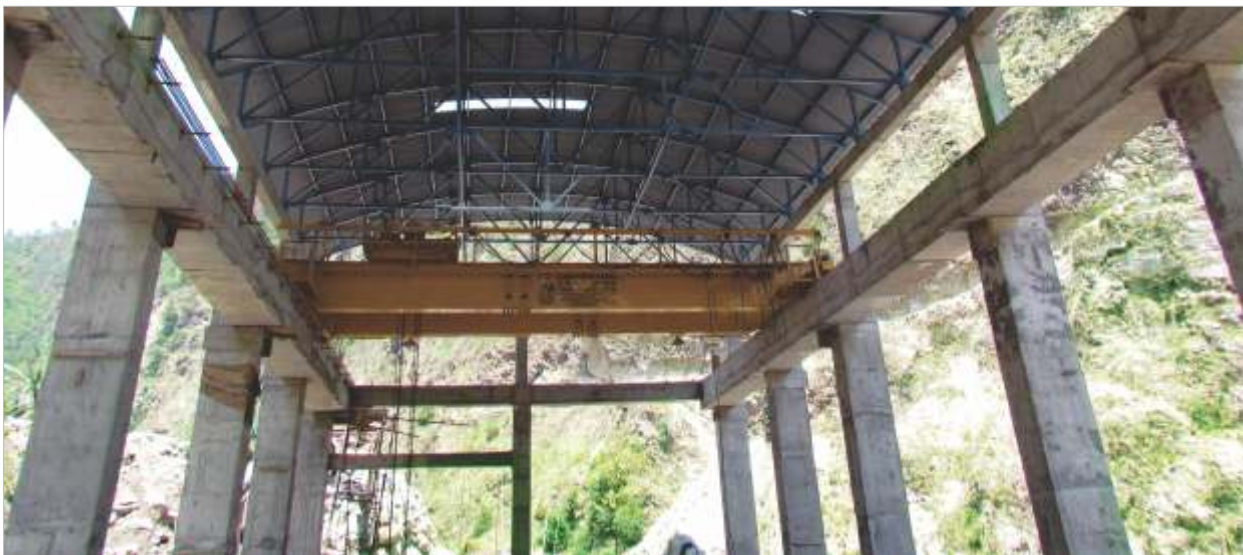
EOT Crane at Power House
